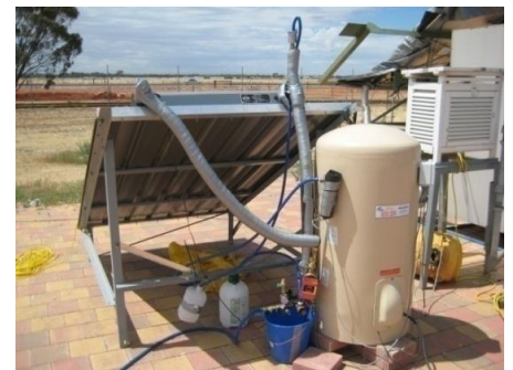
No-load operation test
